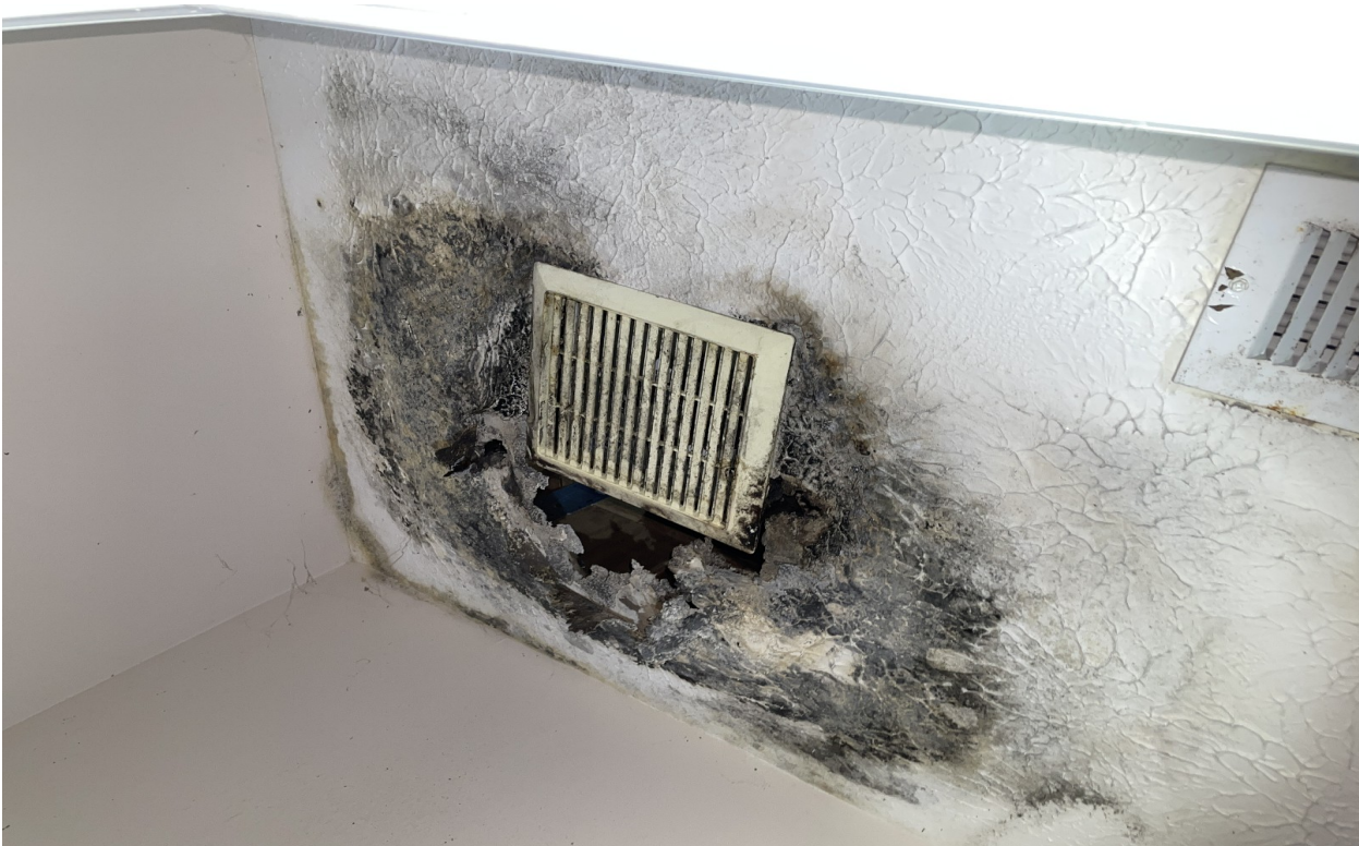
Figure 1-Mold growth on bathroom ceiling
